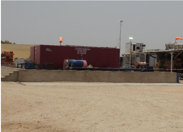
Photograph 4-7: Properly bunded diesel storage area with loading and unloading pad
