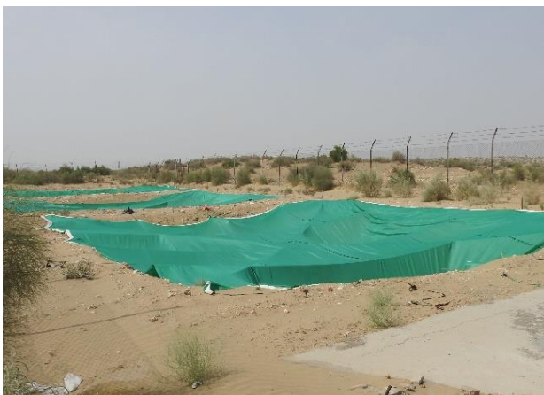
Photograph 4-11: View of a soak pit for disposal of wastewater
