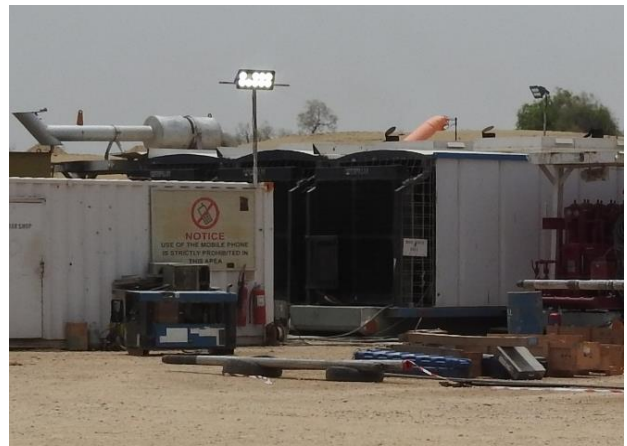
Photograph 4-4: Generators at well site
