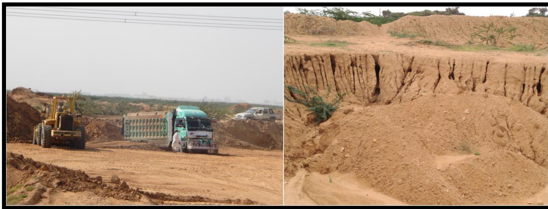
Figure 6-19: Sand Excavation (Left) and Gully Erosion (Right) as Impact of Excavation
