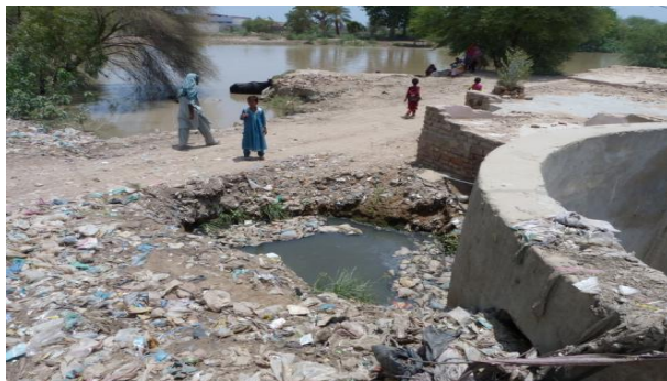
Figure 5-12: Disposal of sewage into Fulleli Canal
